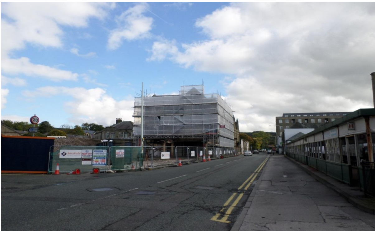
Photo 5 taken September 2017 of Bacup Road Rawtenstall on the left hand side and the bus station on the right hand side.
