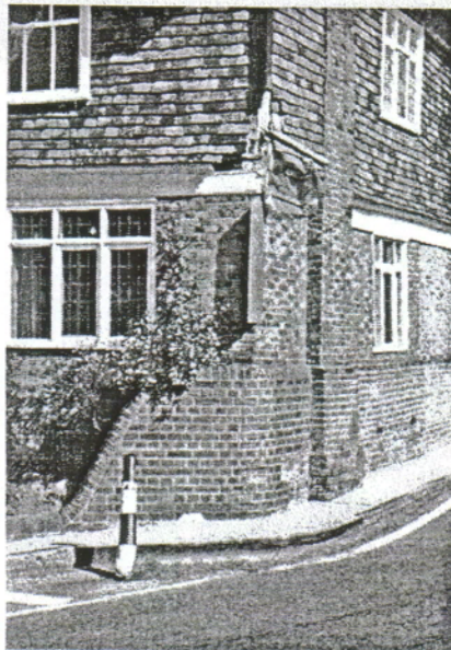
Damage to Buildings
