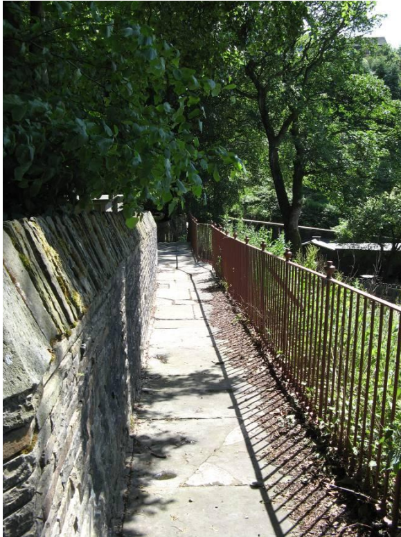
Unpainted railings on edge of churchyard
