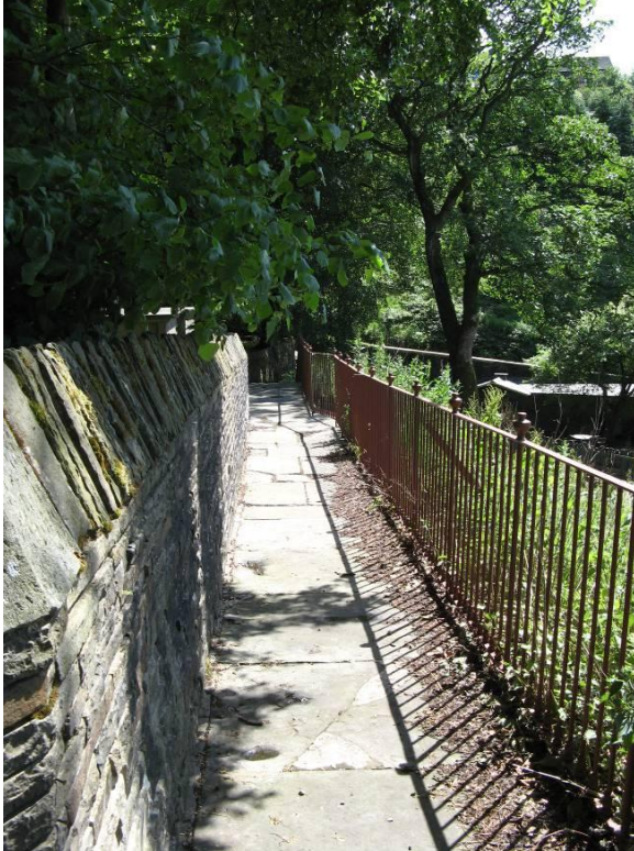
Unpainted railings on edge of churchyard
