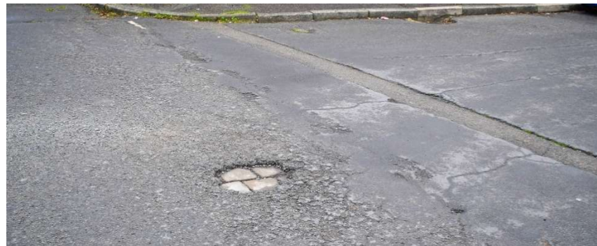
Figure 33 Evidence of earlier cobbles visible through a hole in modern tarmac.
