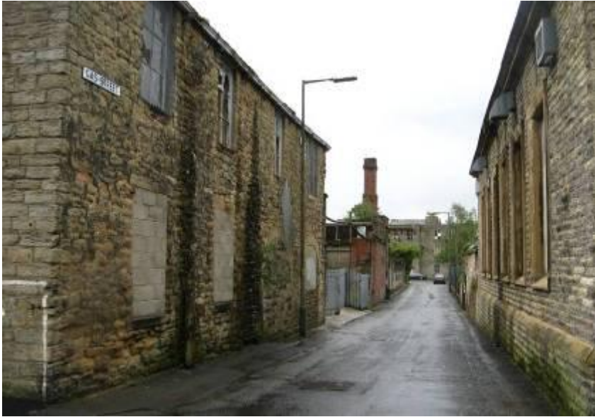
View from Lee Street to the derelict mills beyond the conservation area boundary
