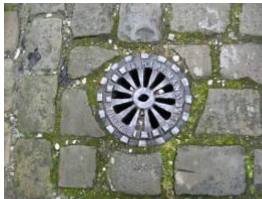
Drain cover in Bank Street
