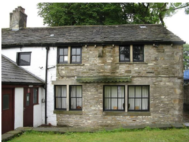
Repairs are need to the CPA Social Club
