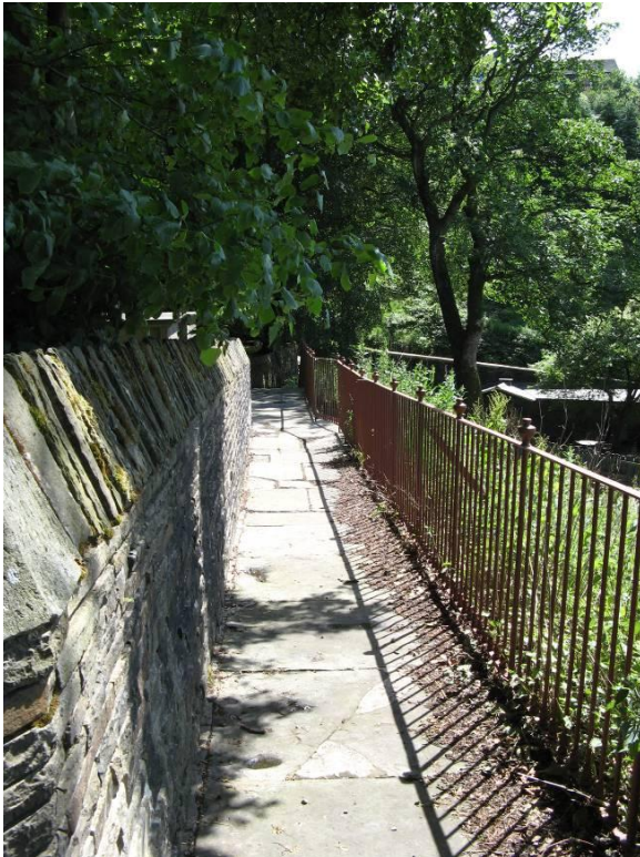
Unpainted railings on edge of churchyard
