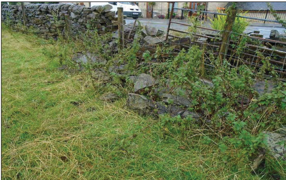
Figure 11: Damaged wall along the western site boundary.
