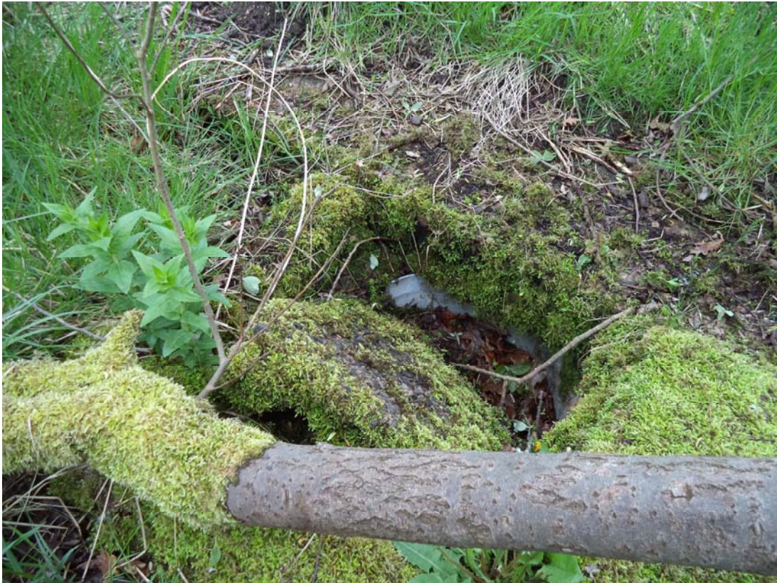
Photograph 9 Relict drainage gully at western slip crest
