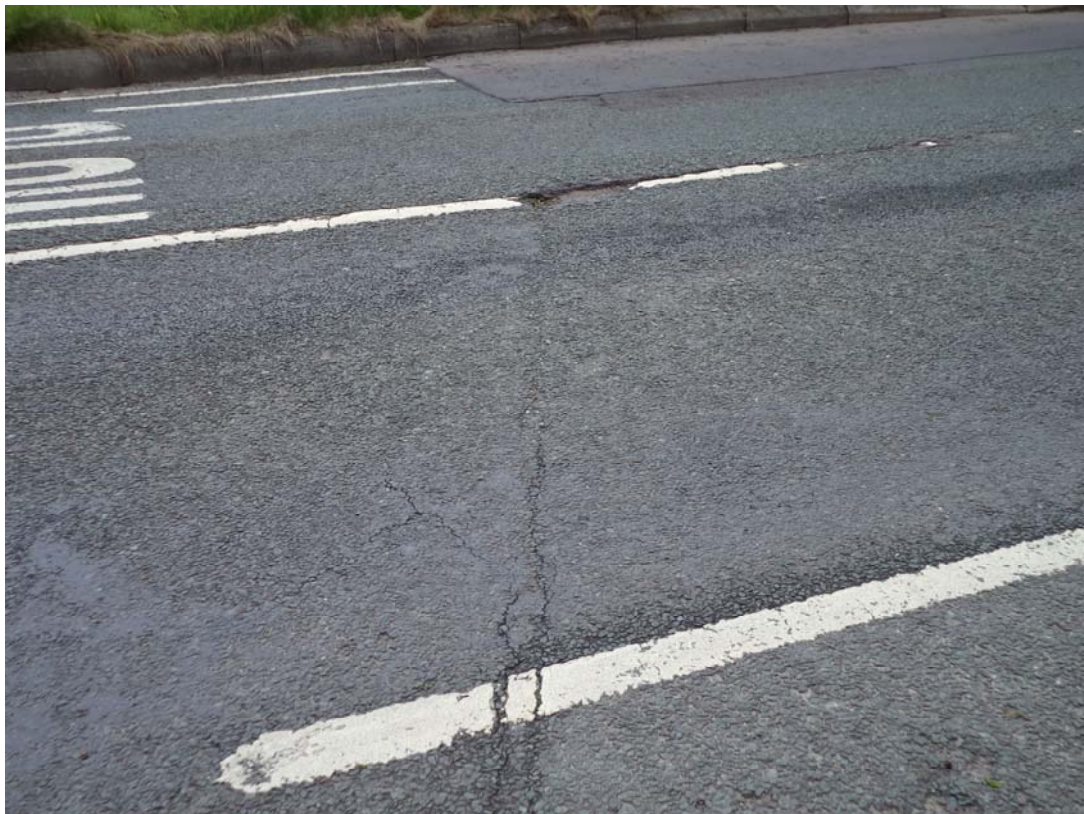
Photograph 22 Damage and repair to road surface to the north of the site on Manchester Road
